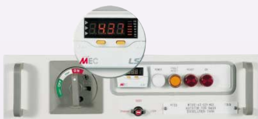
*Fig. (D-EMPR in the MCC unit)
